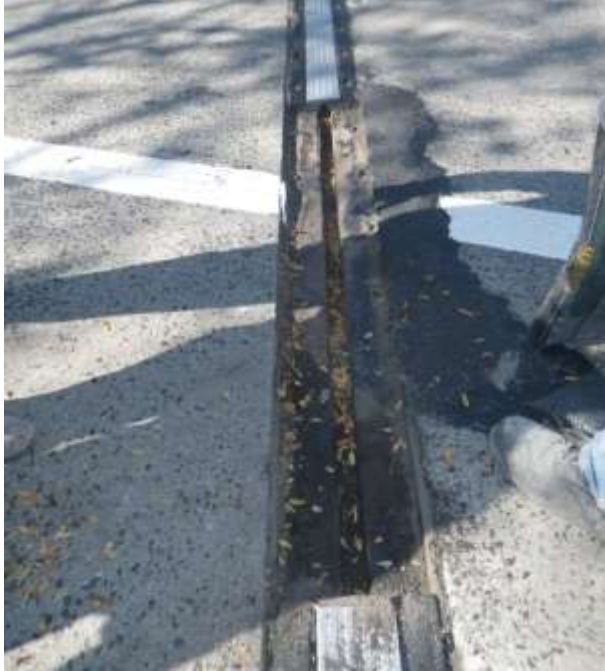
Existing expansion joint after removal of one particularly deteriorated section
