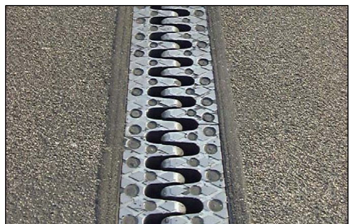
Figure 2: Cantilever finger joint – As installed
