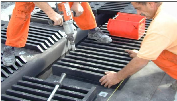
Fig. 5: Positioning and securing of finger plates of a Tensa-Flex joint by hand, on a prepared concrete surface with waterproofing membrane
