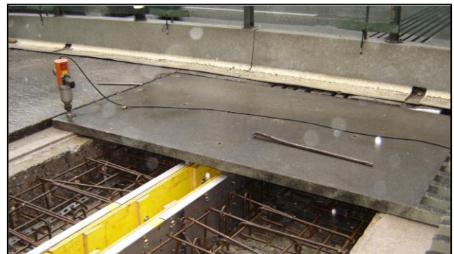
Fig. 6: Placing of Mini-Fly-Over traffic management system to minimise traffic disruption during installation of Tensa-Flex joints
