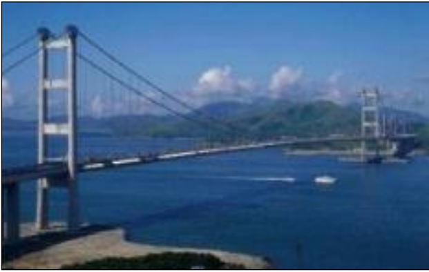
Fig. 7: The Tsing Ma Bridge in Hong Kong – with deck movements facilitated by 25-gap Tensa-Modular expansion joints since 1996
