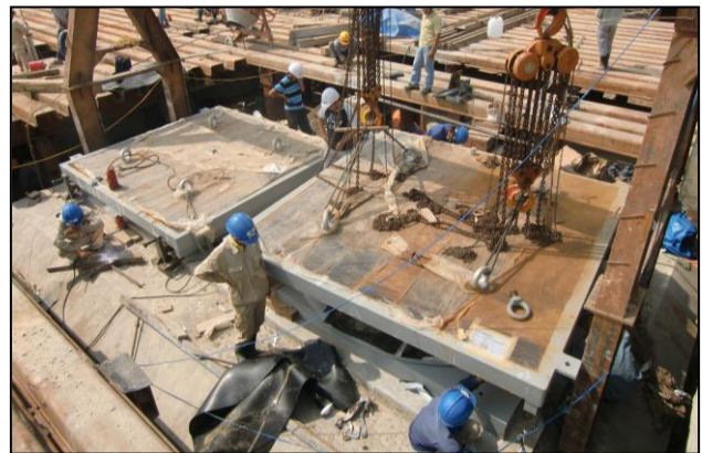
Figure 14: Placing of two enormous guided sliding spherical bearings, side by side, to support the pylon of the Tran Thi Ly Bridge
