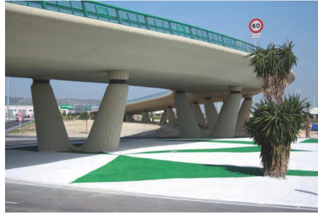
Fig. 2: View of the viaduct from ground level, showing its attractive pier design
