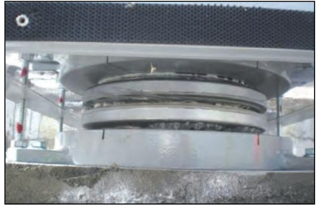
Fig. 16: Free sliding spherical bearing as installed, showing reflection in sliding sheet
