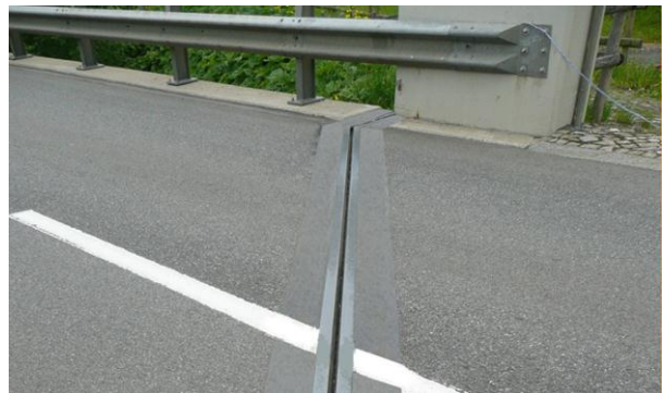
Fig. 10: Single gap joints with anchorage in polymer concrete can be installed diagonally and detailed with horizontal or vertical bends
