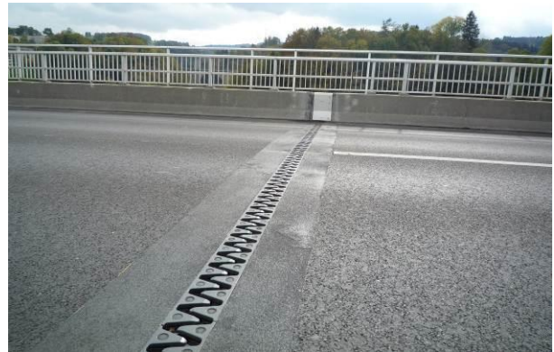
Fig. 16: A single gap joint (of type anchored in polymer concrete) featuring sinus plates
