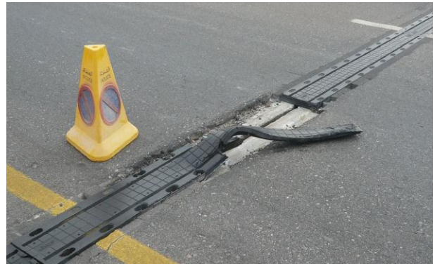
Fig. 3: Alternative types of small movement joint typically offer considerably less strength, durability, reliability and watertightness
