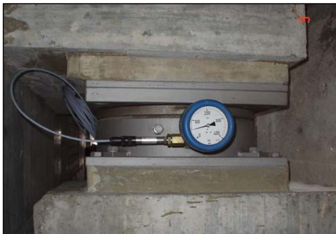
Fig. 10: Load monitoring at a bridge bearing
