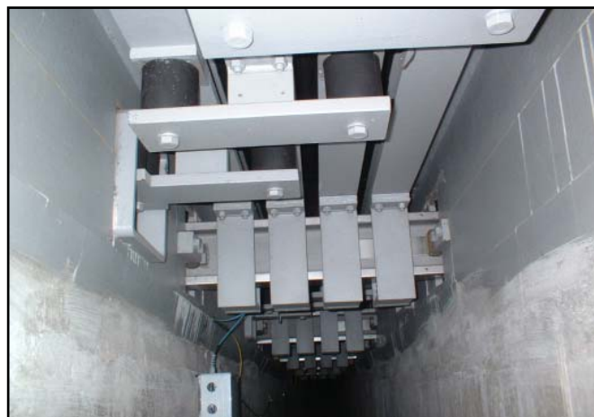
Fig. 11: Movement monitoring sensors at an expansion joint
