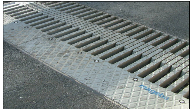
Fig. 4: Sliding finger joint - steel system (Tensa® Finger Type GF) - as installed
