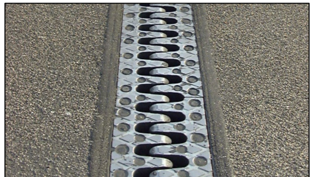
Fig. 2: Cantilever Finger Joint (Tensa ® Finger Type GF) – as installed
