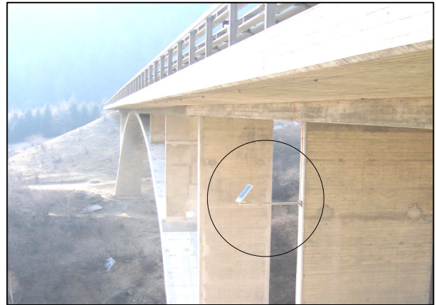
Figure 2: Solar panel of monitoring system
