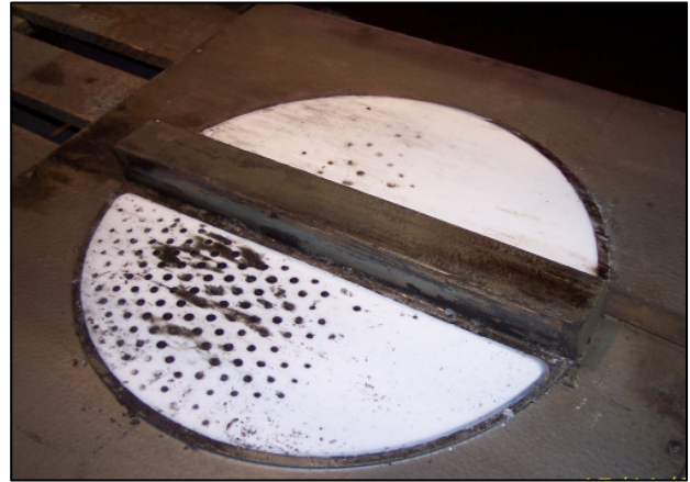
Figure 11: Excessive friction to be investigated
