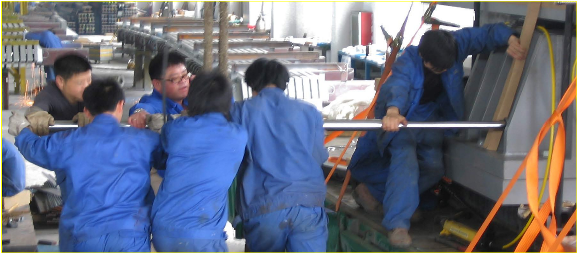
Fig. 5: Fastening of the bolts of the bearings
