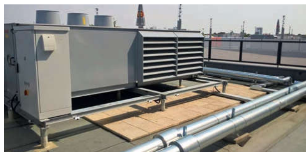
Ventilation plant on the foyer roof with vertical outlet ducts
