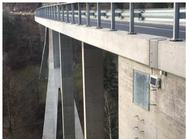
Figure 7. Abutment at one end of bridge, showing access hatch to internal area with bridge bearings
