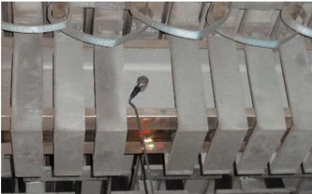
Figure 16. An accelerometer at the location of a temporarily removed stirrup during fault simulation and measurement of resulting vibrations and modal analysis
