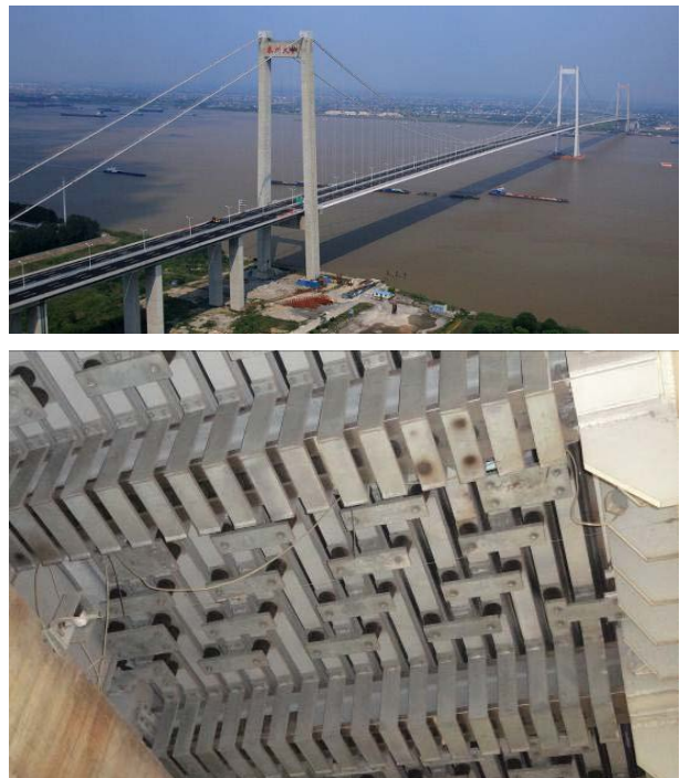
Figure 15. The Taizhou Yangtze River Bridge and one of its expansion joints, viewed from below
