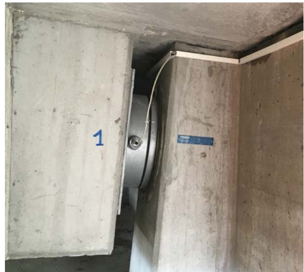
Figure 9. One of the new vertically oriented bearings at one abutment, retrofitted to provide longitudinal fixity to the deck at this end
