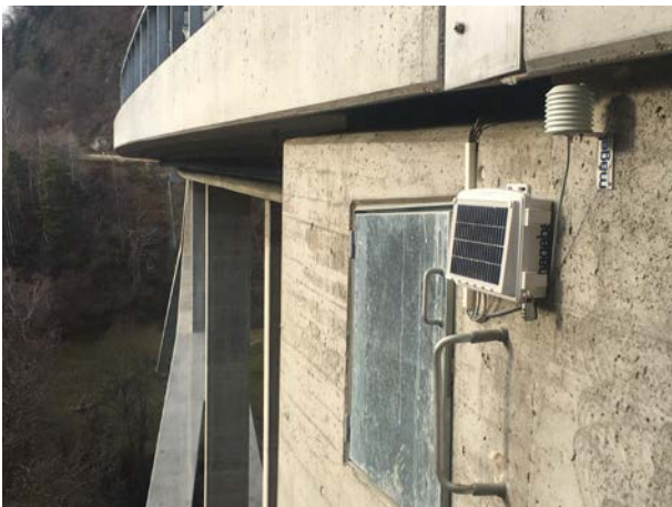
Figure 8. The heart of the SHM system, installed externally at one abutment, complete with integrated solar panel on its cover for power supply and a separate weather sensor
