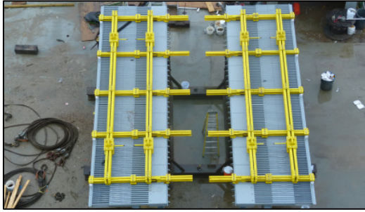
Figure 15. View of two joints from above after adjustment of pre-setting on site.
