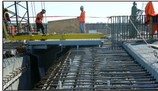
Figure 19. View of Axis 3E after positioning of one of its two joints.
