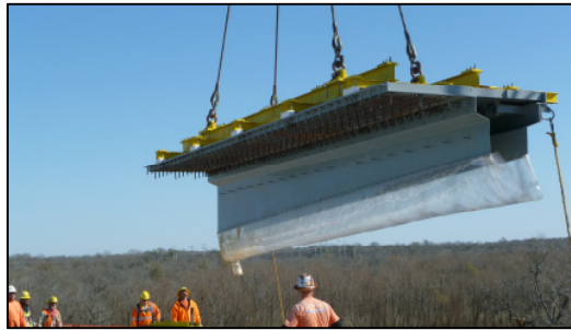
Figure 18. Lifting into position of a fully assembled expansion joint at Axis 3E.
