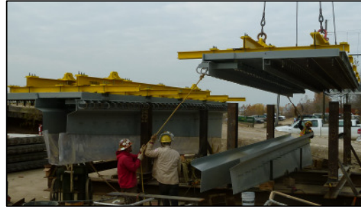
Figure 16. Connection of drainage channels to joints after placing on a support frame.
