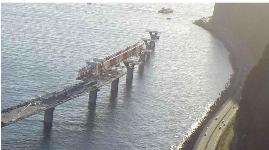
Figure 5. Placing of precast segments in the viaduct as it extends along the shoreline
