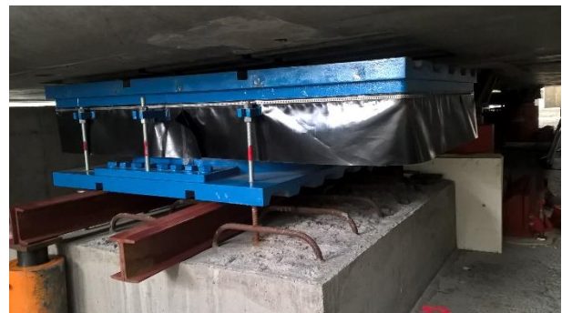
Figure 25. Installation of a bearing on site, before concreting/grouting of connections to main structures above and below the bearing
