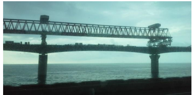
Figure 4. View of the equipment used to extend the superstructure, segment by segment
