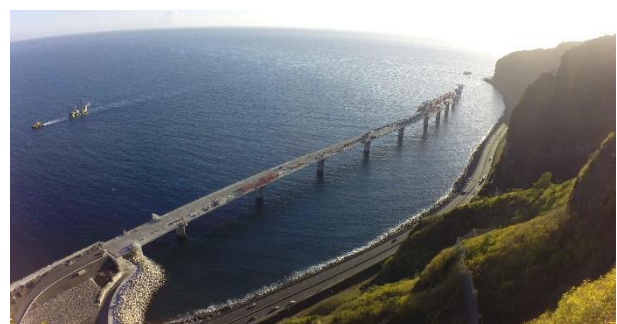
Figure 1. Part of the "Nouvelle Route du Littoral" during construction on a viaduct along the shoreline of La Reunion in the Indian Ocean
