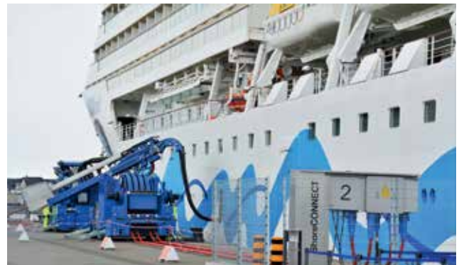
Cable Management System (CMS) at Berth 8
