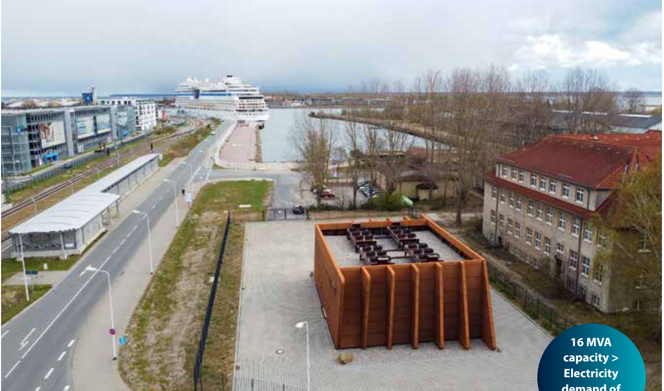
View of onshore power supply facility and adjacent berth
