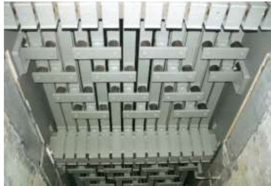
Figure 4. An installed Tensa-Modular expansion joint, viewed from below.
