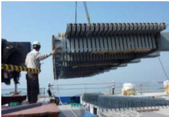
Figure 3. Installation of a Tensa-Modular expansion joint on a bridge with a concrete deck.
