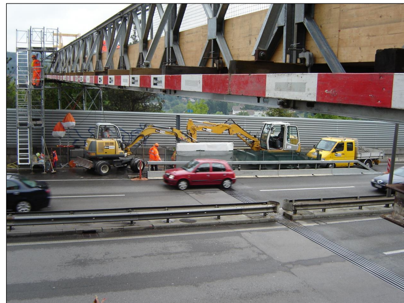
Step 1: One lane was closed during a weekend (when traffic was light)
