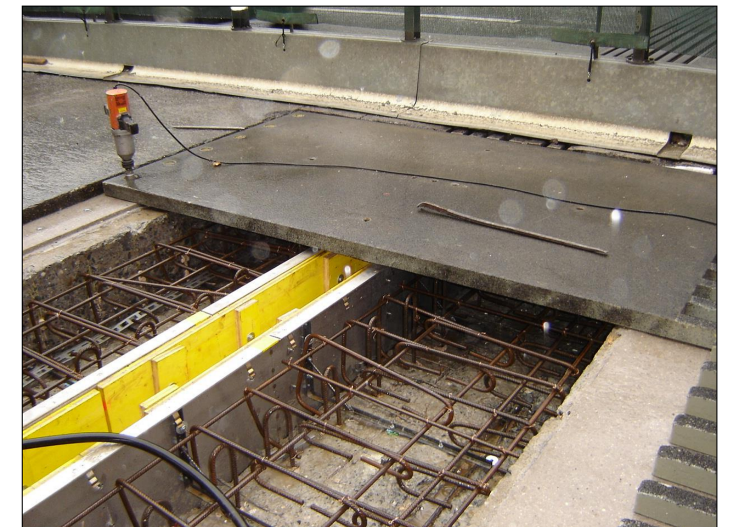
Step 4: Mini-Fly-Over finger plates were then placed and secured, to carry traffic
