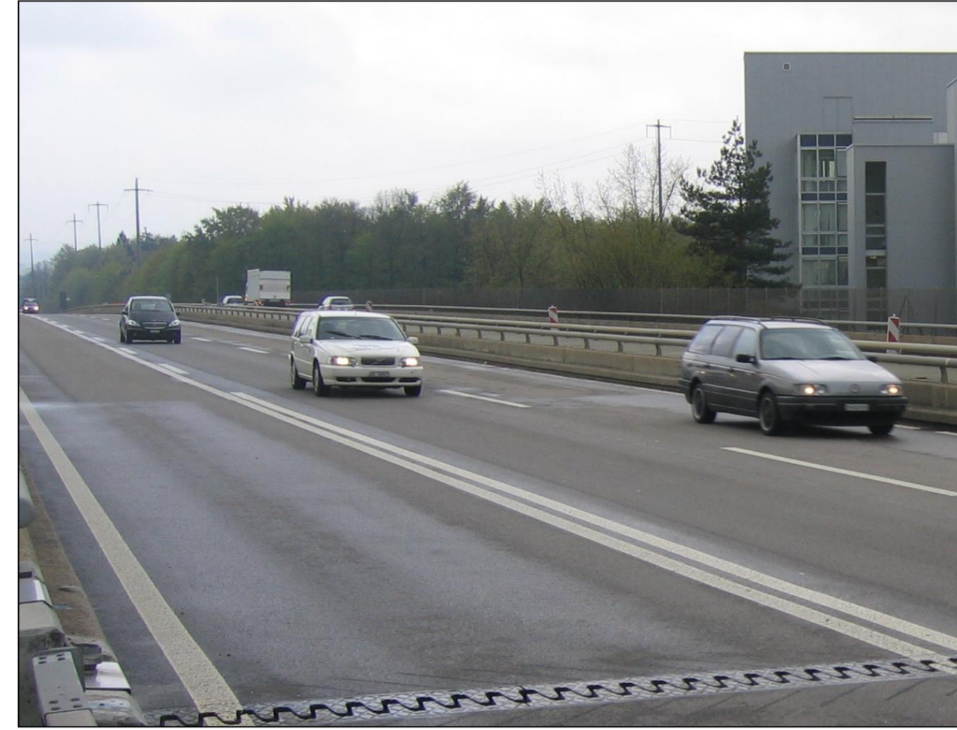
Such disruption can be caused during replacement of bridge expansion joints
