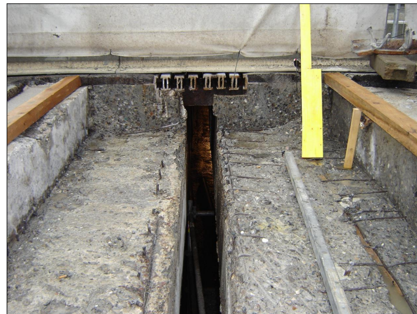
Step 2: This allowed the existing joint to be removed without impacting on traffic
