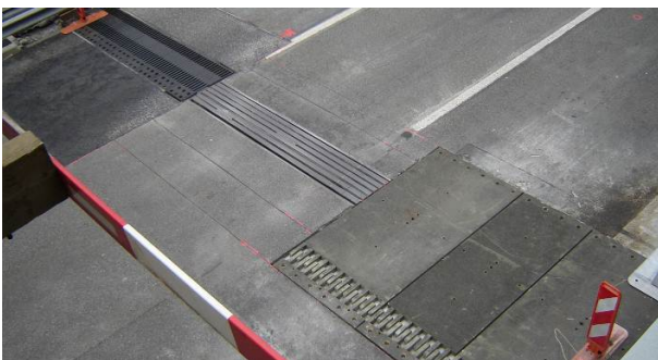
Figure 7. Three-lane carriageway during replacement of old modular joint (centre) with new Tensa-Flex joint (left) using Mini-Fly-Over (right)
