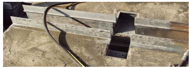
Figure 8. View of retained substructure following removal of the dynamically loaded mechanical part of the old modular joint
