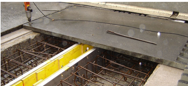
Figure 6. The Mini-Fly-Over system can be used to allow traffic to cross the site during the day, making even this lane open to traffic when needed
