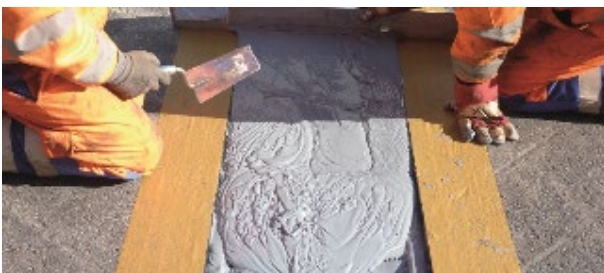
Figure 3. Installation of this low-depth joint on an existing structure typically requires no breaking out of concrete and can be carried out lane by lane
