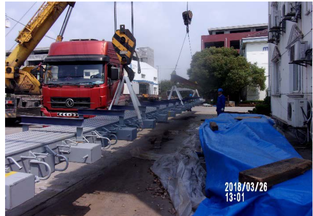
Figure 9. Loading of joints with lengths of up to 25m for transport from the factory in Shanghai
