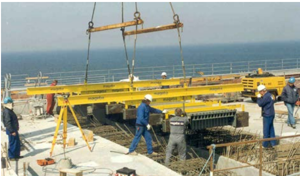
Figure 13. Installation beams across the top of the joint enable it to be precisely positioned and height-adjusted using hydraulic jacks under the ends of the beams at each side of the bridge gap
