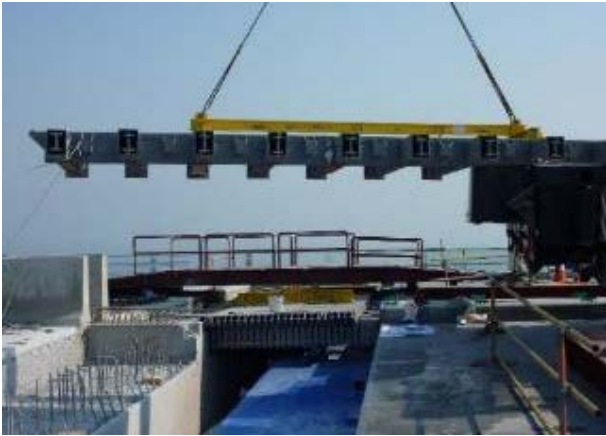
Figure 12. Before lifting a joint into the blockout in a bridge deck, using load-spreading beams as necessary, the blockout must be suitably prepared
