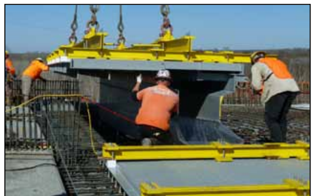
Fig. 22: Lifting into position of the second expansion joint at one bridge axis
