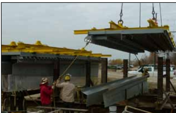
Fig. 21: Connection of drainage channels to joints after placing on a support frame
