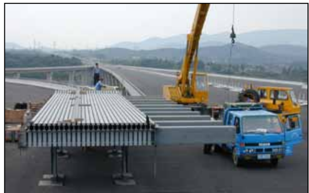
Fig. 17: Assembly on site of world-record 27-gap modular joints for the Run Yang Bridge, China 2004
