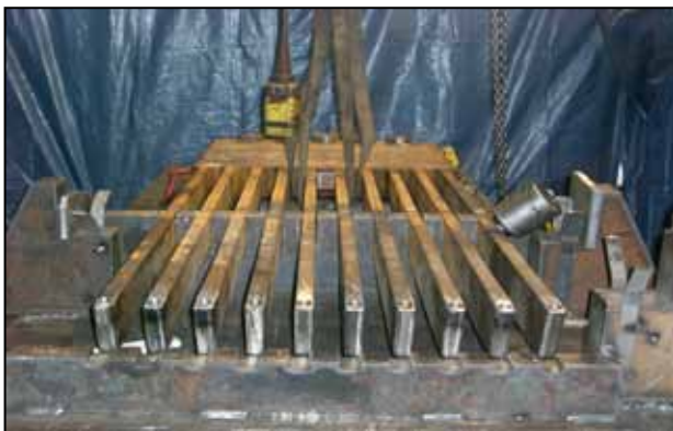
Fig. 19: Mechanical straightening of the fingers of a sliding finger plate
