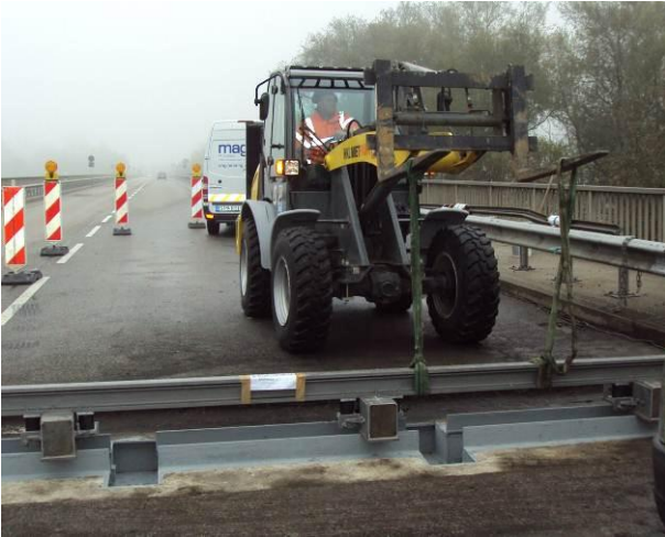
Fig. 11: Lifting in of the new structure, consisting of a lamella beam and connected support bars, complete with boxes
