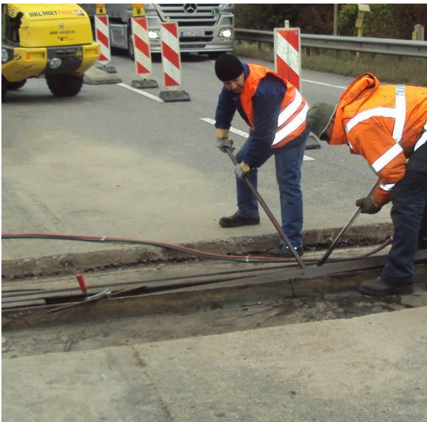
Fig. 8: Removal of the lamella beams of the old joint, following removal of asphalt
