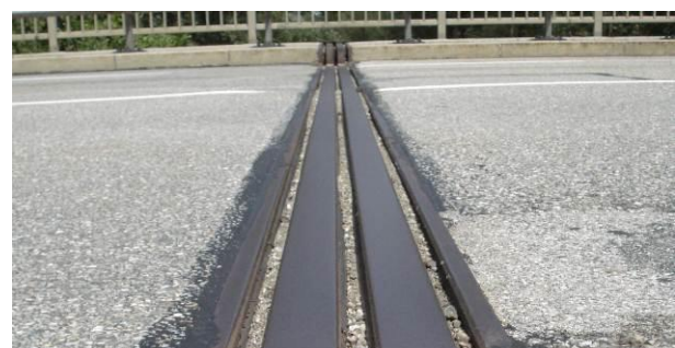
Fig. 7: The existing 3-gap modular joint
