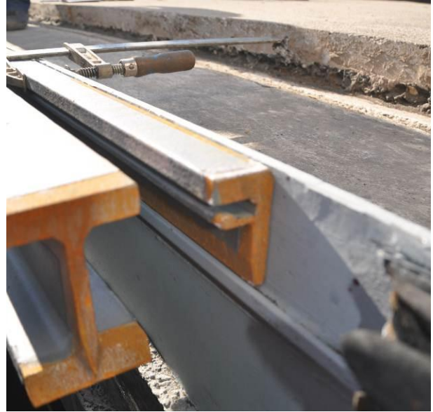
Fig. 16: Completion of a new edge profile with the addition of a new part into which the edge of an elastomeric seal will be inserted
