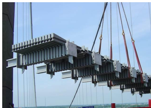
Fig. 3: A modular joint during lifting into position on the Lillebaelt Bridge, Denmark
