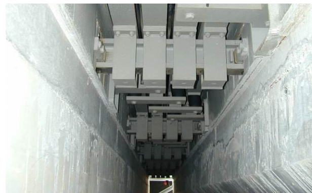
Fig. 6: View of an installed 5-gap modular joint, from beneath
