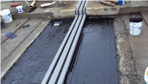
Fig. 19: Application of waterproofing to bridge deck at each side of the new joint
