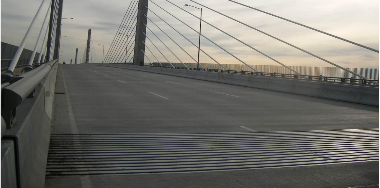
Fig. 1: A large modular expansion joint at one end of the deck of a cable stayed bridge
