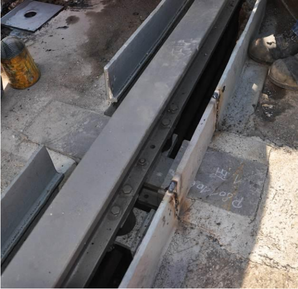
Fig. 15: The vertical plate of the edge profile at one side of the joint has been welded back in place
