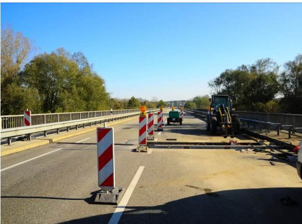
Fig. 21: Phased approach to further reduce the impact on traffic – with work carried out one lane at a time
