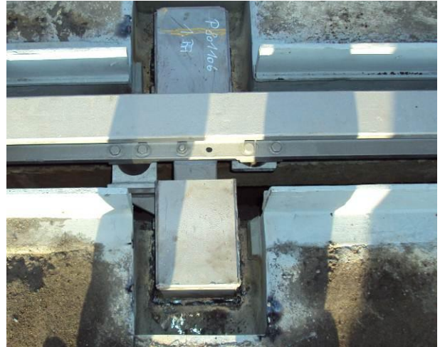
Fig. 12: View of a support bar box of the new joint, placed inside the larger support bar box of the old joint and welded all around
