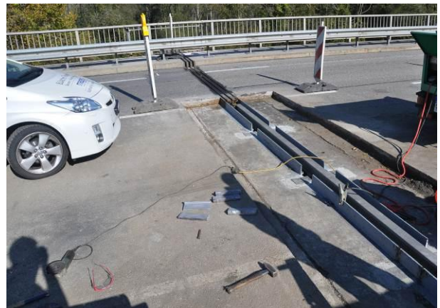
Fig. 14: View of joint following securing in place, before re-instatement of edge profiles
