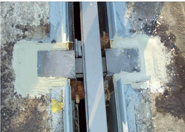
Fig. 13: View of one new support bar and its boxes, following placing of mortar to fill out the voids between new and old boxes
