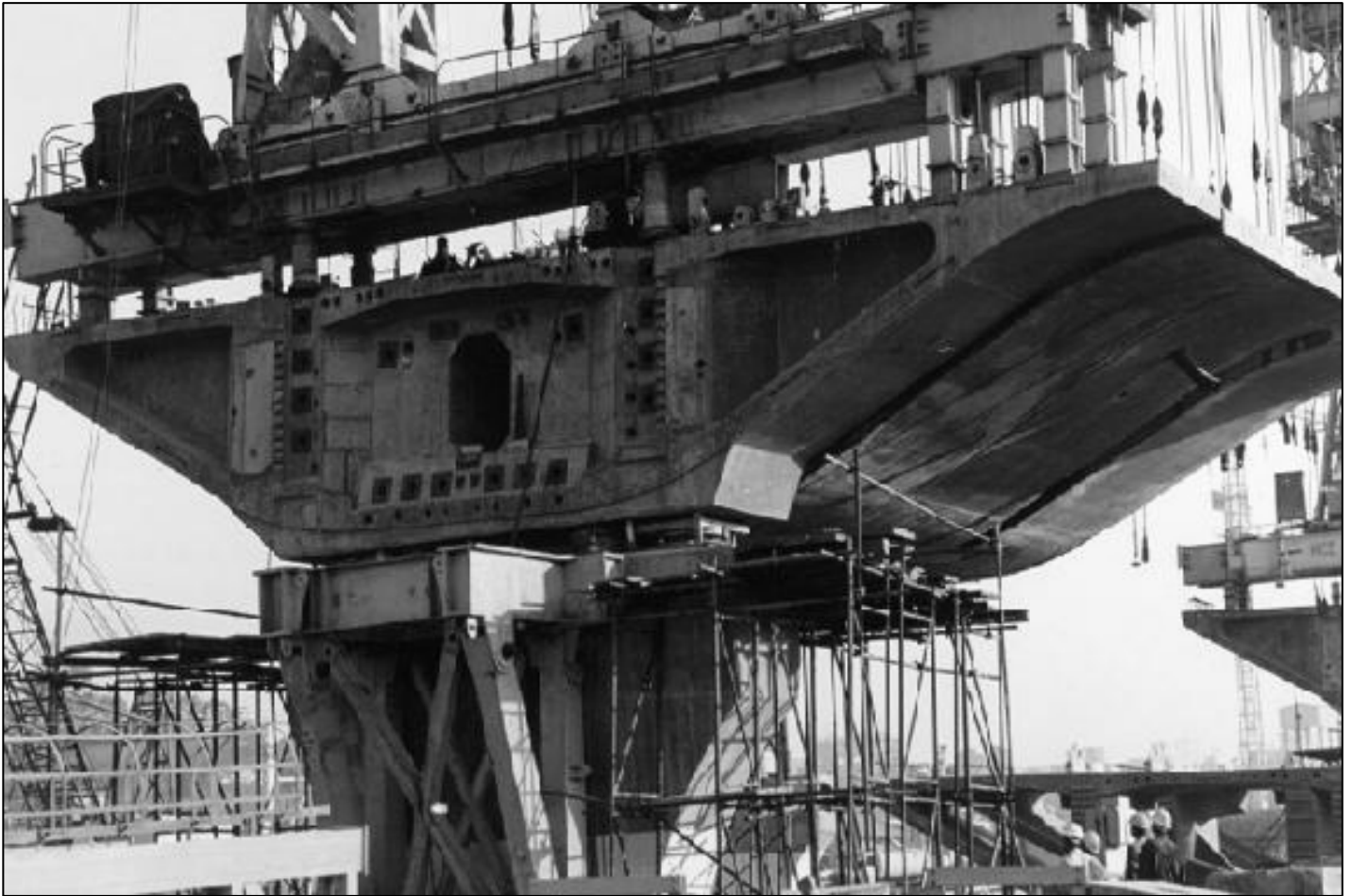
Figure 5. Erection of bridge segment over disc bearing in Bandra Worli Sea Link
