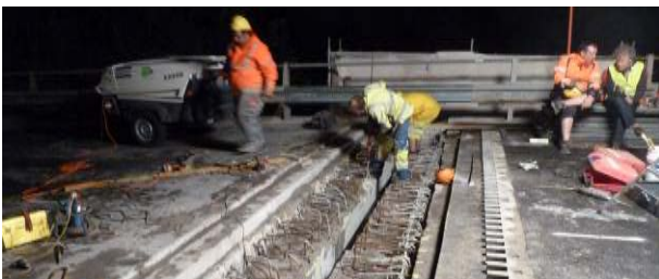
Figure 35. Final preparation of recess prior to lifting in of a new cantilever finger joint
