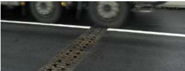
Figure 28. A Tensa®Finger Type RSFD expansion joint in service on a bridge
