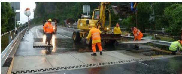
Figure 34. Removal of Mini-Fly-Over at start of a work shift to allow recess preparation to proceed
