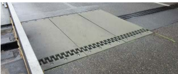
Figure 24. Mini-Fly-Over in place in centre lane while outside lane closed for replacement works
