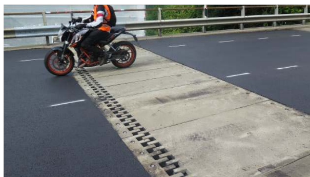
Figure 2. Traffic can flow freely during peak hours, with Mini-Fly-Over (in this case raised above normal surface) spanning the construction area
