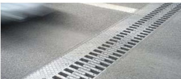
Figure 19. A Tensa®Finger (Type GF) sliding finger joint in service
