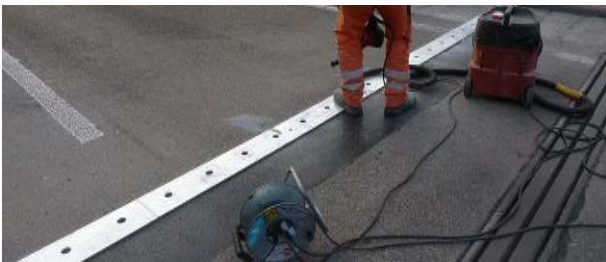
Figure 32. Drilling of holes (using template) in polymer concrete strips for Mini-Fly-Over anchors
