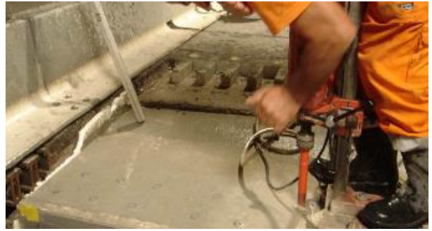
Figure 13. By Wednesday evening, concrete cured sufficiently to drill anchor holes and place dowels
