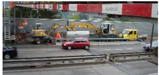
Figure 6. Start of work on first Friday evening, with one lane closed until Monday morning
