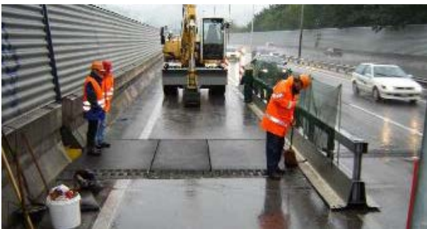
Figure 11. Early on Monday morning, site cleared to allow lane to be re-opened to traffic
