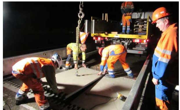
Figure 25. Removal of Mini-Fly-Over in one lane at start of a weekend shift
