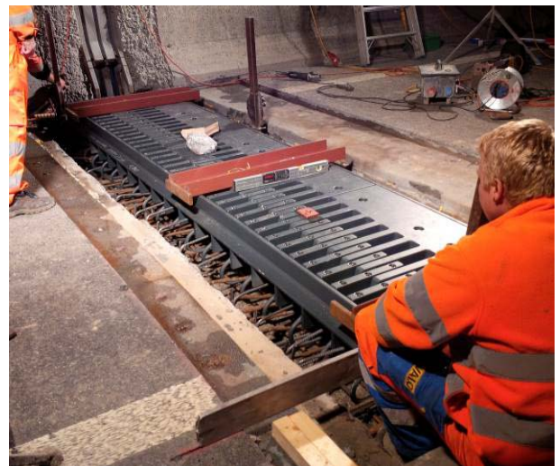
Figure 27. Levelling of new finger joint prior to concreting and completion of connecting road surfacing
