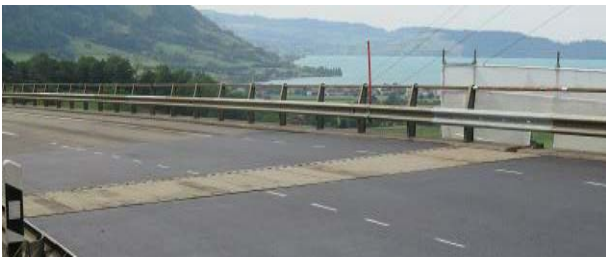
Figure 33. Following anchoring of Mini-Fly-Over in place, road surface temporarily tapered at each side with new asphalt to suit level of plates
