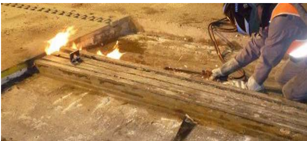
Figure 23. Removal of joint in second lane for placing of Mini-Fly-Over during second weekend
