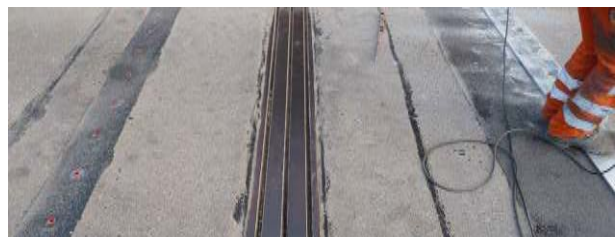
Figure 31. The existing expansion joint prior to removal, with polymer concrete strips (darker colour) cast at each side to support Mini-Fly-Over
