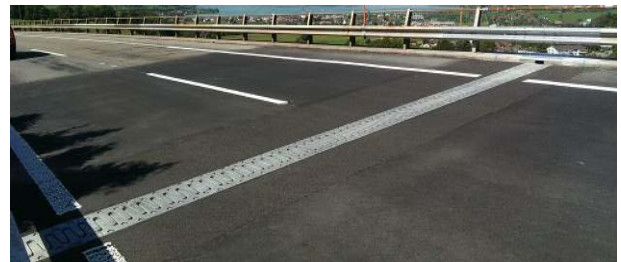
Figure 37. Fully installed cantilever finger joint following concreting in place, and removal of tapered ramps and re-asphalting at each side
