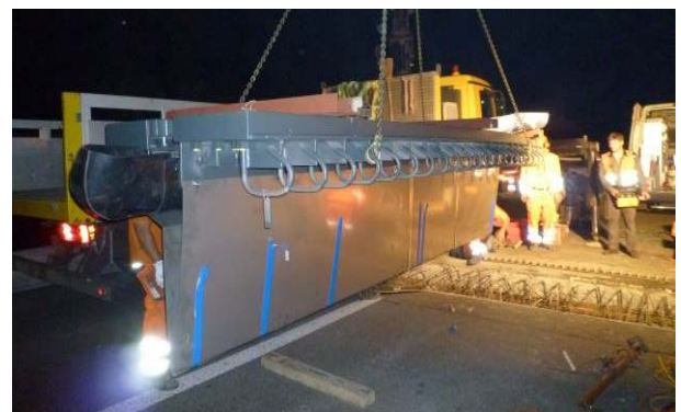
Figure 26. Lifting in of the new finger joint in the first lane during the third weekend
