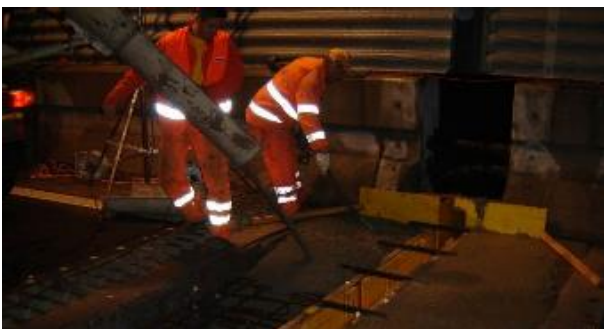
Figure 12. On Monday night, lane closed to traffic again, Mini-Fly-Over removed and concrete placed
