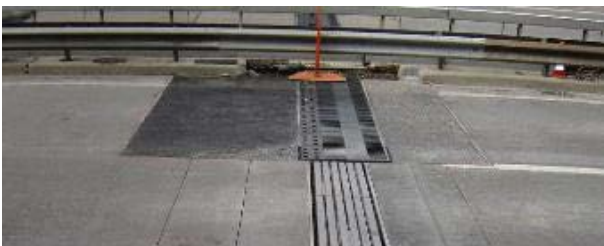
Figure 18. After one week, with road newly asphalted, first phase finished and joint in service
