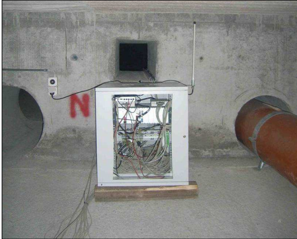
Fig. 5: Installation of Robo ® Control computer
