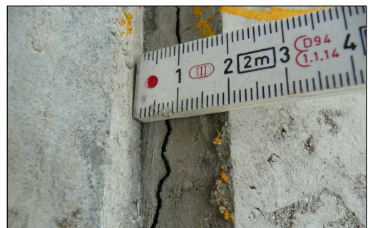
Fig. 2: Detail of an observed crack
