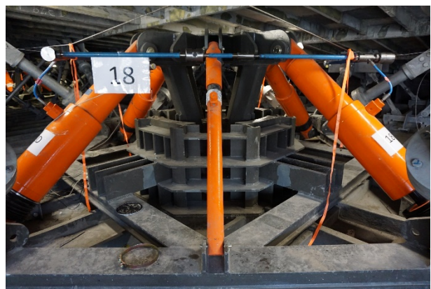
Figure 10. Vibrations at each of the 30 column heads are damped by two Reston-SA shock absorbers and four Reston-SP spring devices
