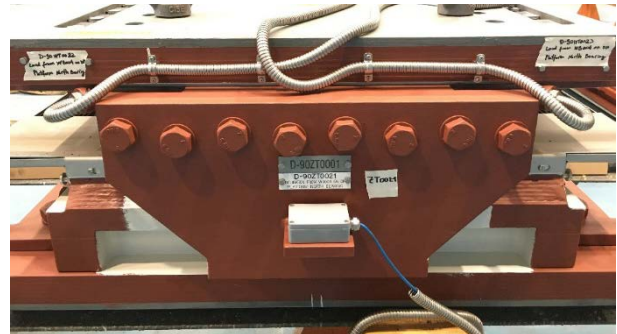
Figure 6. Inclinometer on side of a bearing
