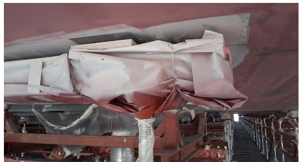
Figure 14. After seven days of injection, the roof canopy lifts off the scaffolding
