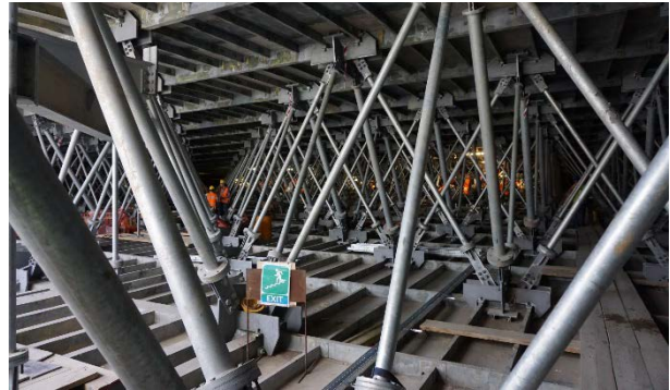
Figure 9. View inside the roof canopy, showing truss structure between top and bottom skins
