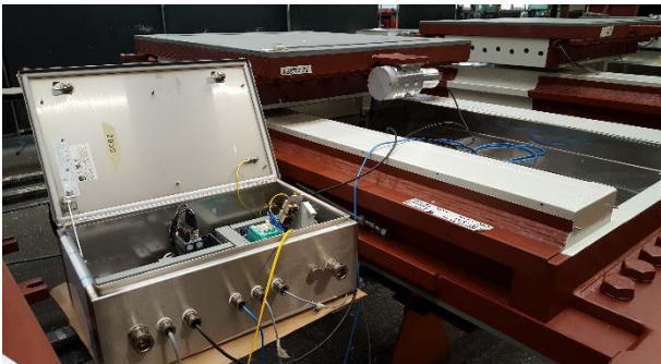
Figure 4. Installation of sensors on a sliding bearing with connection to Signal Conversion Box
