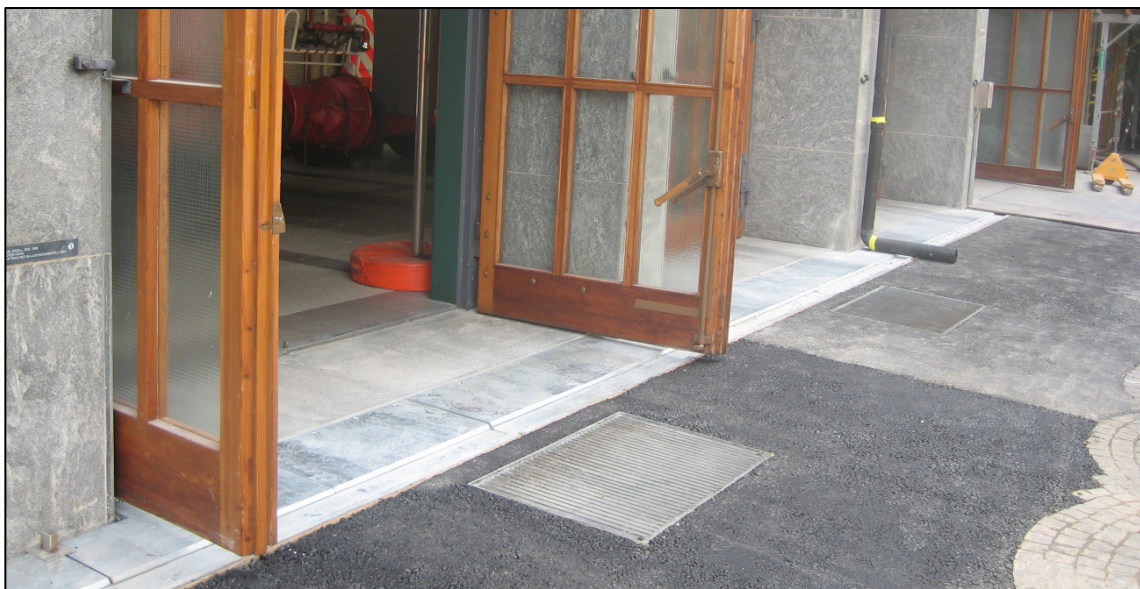
Figure 11. Vehicle exit point after completion of works, showing new stainless steel expansion joint
