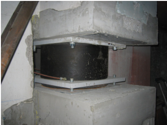
Figure 5. Seismic bearing installed beneath pillar at perimeter of building
