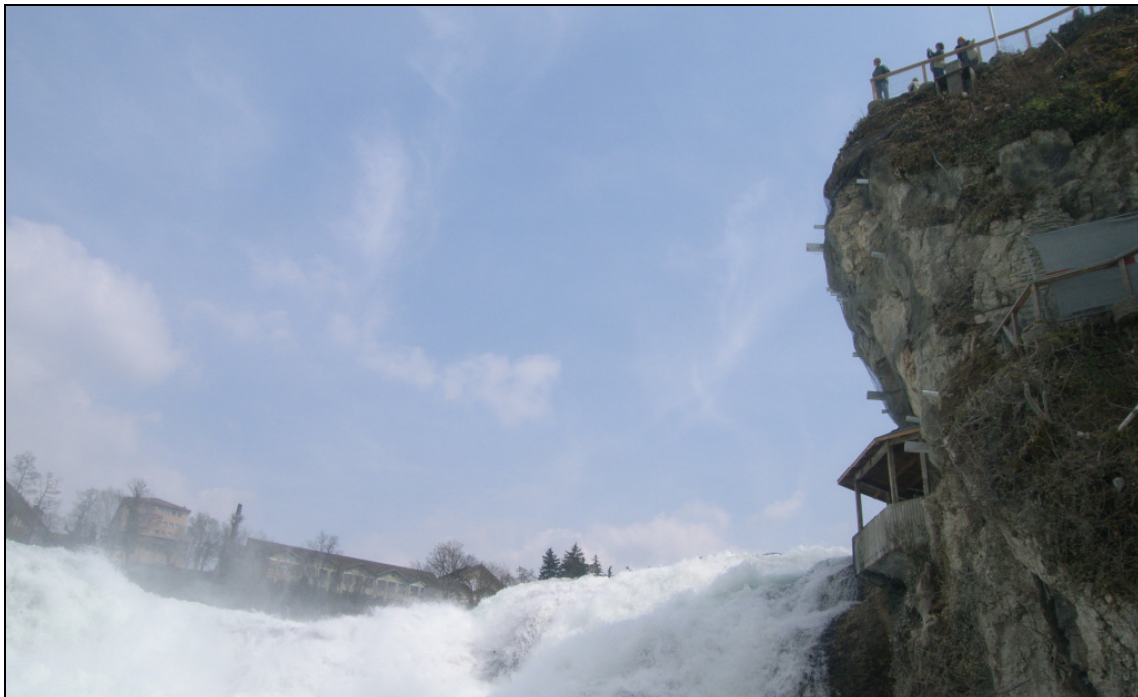
Figure 7. Rock wall of main interest with public terrace on top, stabilised with 11 new rock anchors.
