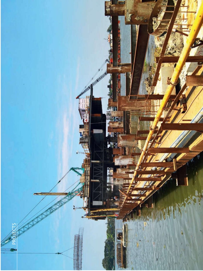
Piling rig at work during construction of Cochin's new ship repair facility
