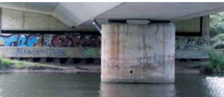
ASR-damaged central pier of the Spree Bridge
