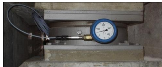
Figure 9. Load monitoring at Ponte Nanin bearing.
