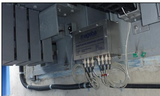
Figure 1. Bridge computer of a monitoring system, with connections to all measurement sensors.
